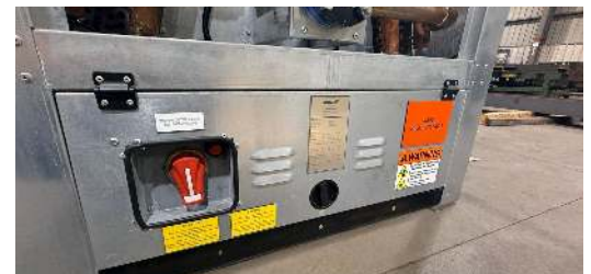
SERVICE / ACCESS VIEW Power, controls, and disconnect access
